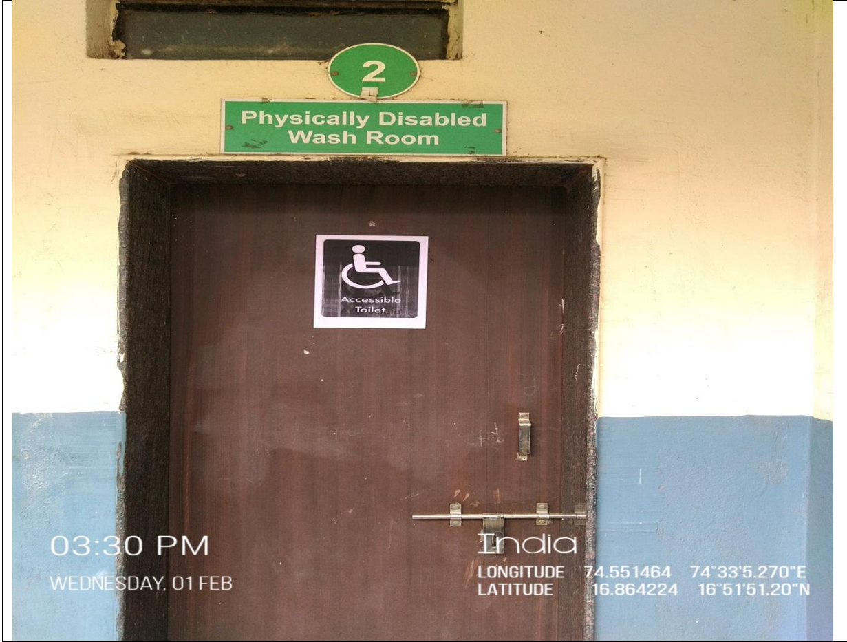
Disabled – friendly washrooms
