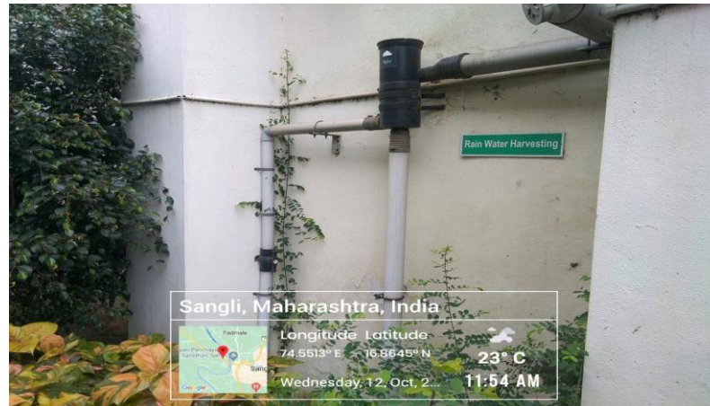
Rain water collection pipe
