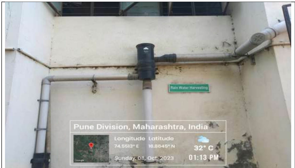
1. Rain water harvesting structures
